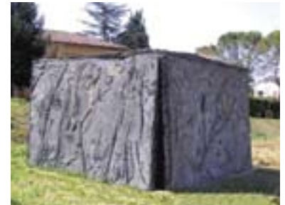
Sub-station at Santa Lucia (designed by G. Spagnulo)
